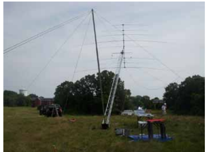
Tower being raised at Medfield 2012 WRTC test station. 40' Rohn 25 tower supported beam and inverted vees/dipoles
